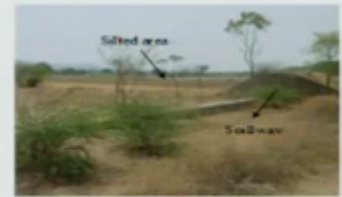
4. Tank spillway and silted area
