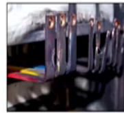
Busbar after Shorting with nearby Busbars. Source: Shutterstock
