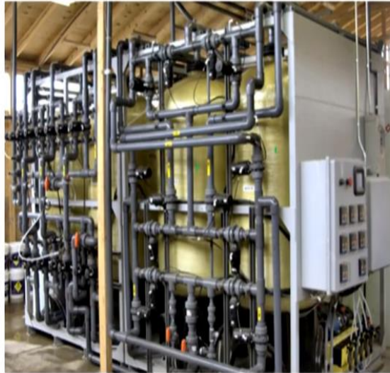
Multicolumn ion exchange system
