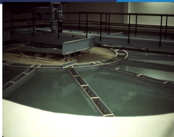
Upflow solids contact tank with radial weirs
