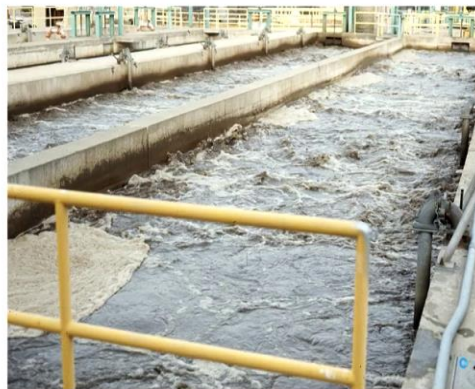
Aeration tanks. Note Nocardia foam at left in foreground.
