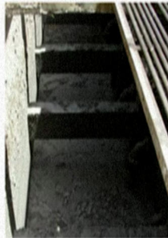
Primary sludge tank
