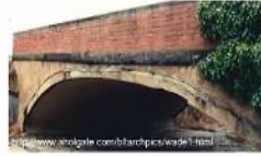
Wade Street Monitor Arch Bridge, Bendigo The arch of Wade St Bridge, Bendigo (1901) has become almost flat in the centre. Creep in the concrete is probably the major factor.
