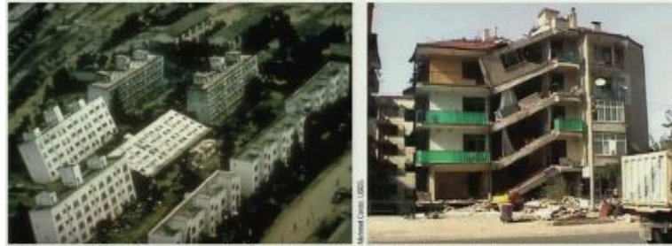
A. These strong buildings in Niigata, Japan, remained intact during the 1964 earthquake but fell over when the sediments below them liquefied. B. Liquefaction of the foundation under the left side of this building during the August 17, 1999, earthquake in Izmit, Turkey, caused settling of the left section and destruction of the middle section.
